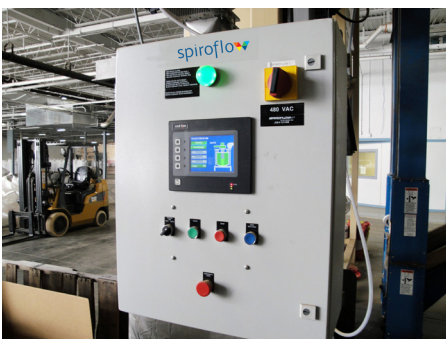
Bulk bag filler gain-in-weight control panel
