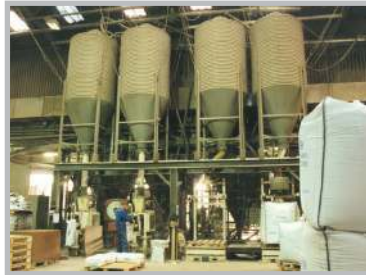
Filling materials in bulk bags and 50 lb (25kg) bags in a minerals processing plant
